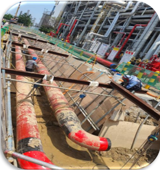
Field Run Piping
