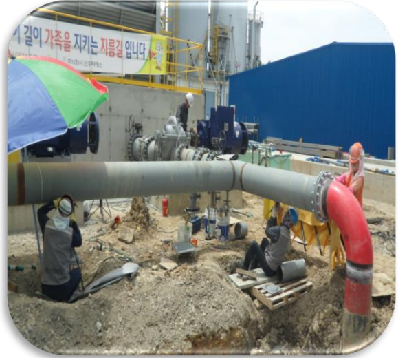
Field Run Piping
