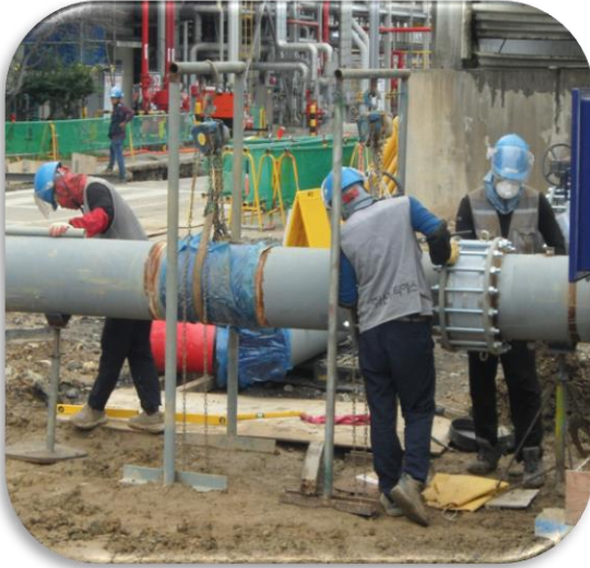
Field Run Piping
